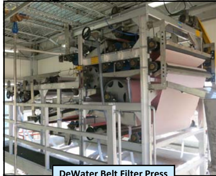
DeWater Belt Filter Press
