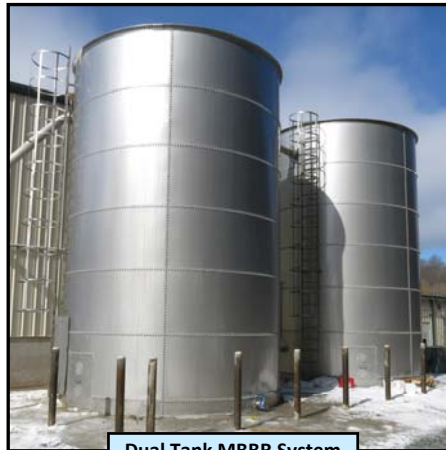
Dual Tank MBBR System
