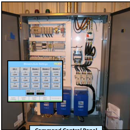
Command Control Panel
