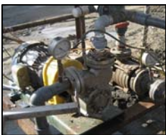
Pump & Control Nightmare
