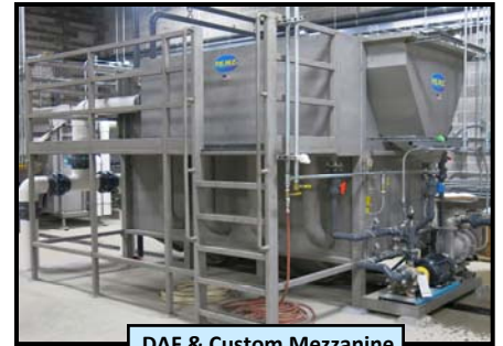
DAF & Custom Mezzanine
